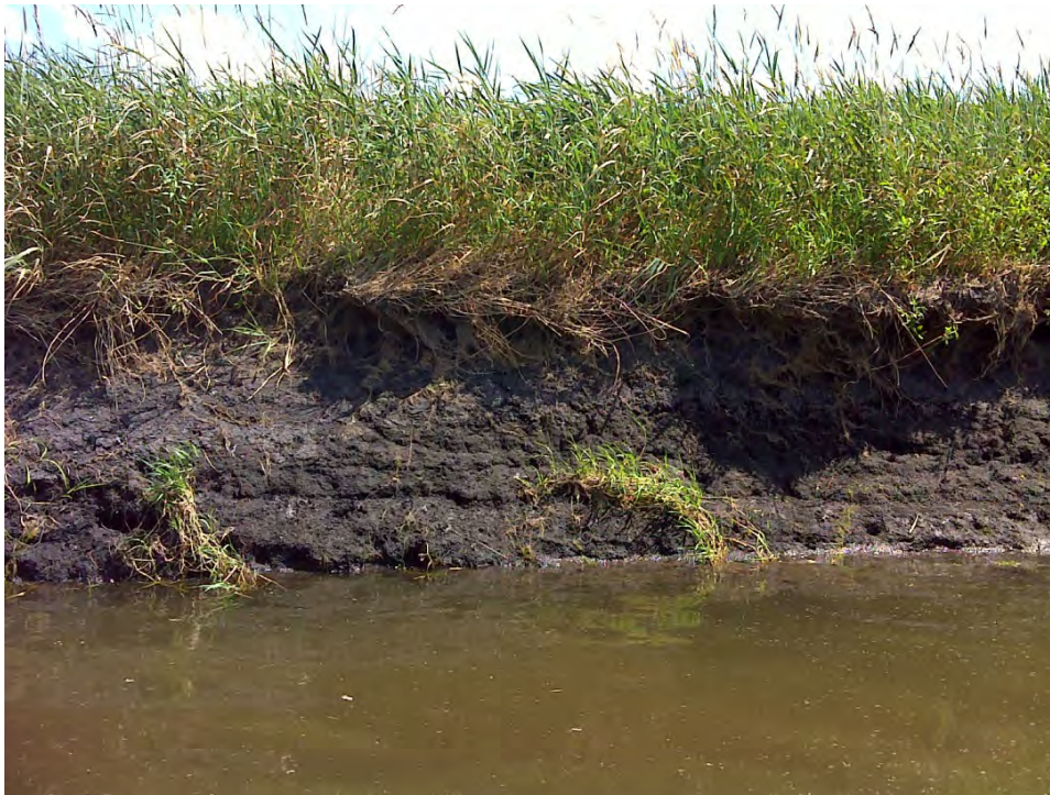
Figure 26. Eroded bank on the Little Sioux River near 11MS010
