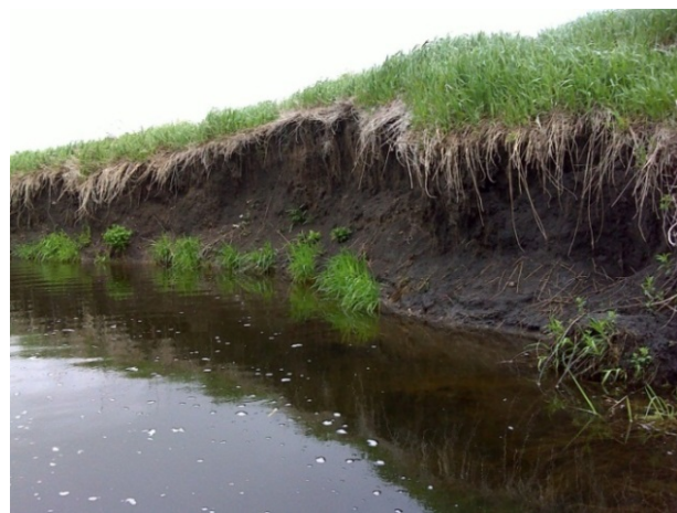
Figure 122: Bank erosion at 11MS113 along Unnamed Creek (10170204-571)
