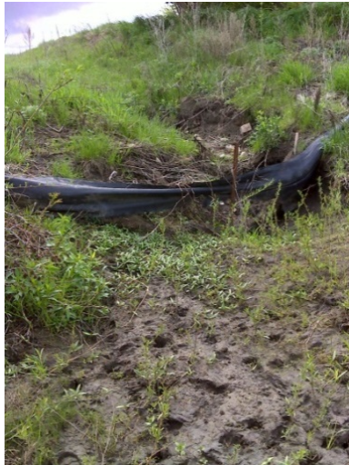
Figure 95: Poor silt fence installation at 11MS003 along the Rock River
