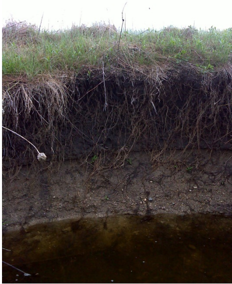
Figure 117: Eroded bank at site 11MS096 along Unnamed Creek (10170204-589)
