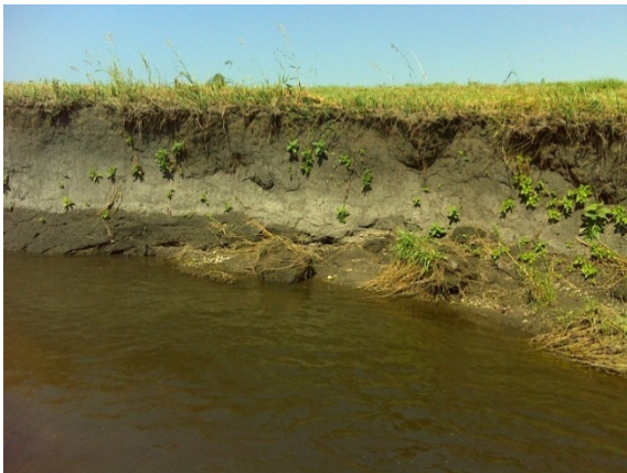
Figure 82: Eroded bank at 11MS047 along Little Rock River (10170204-512)
