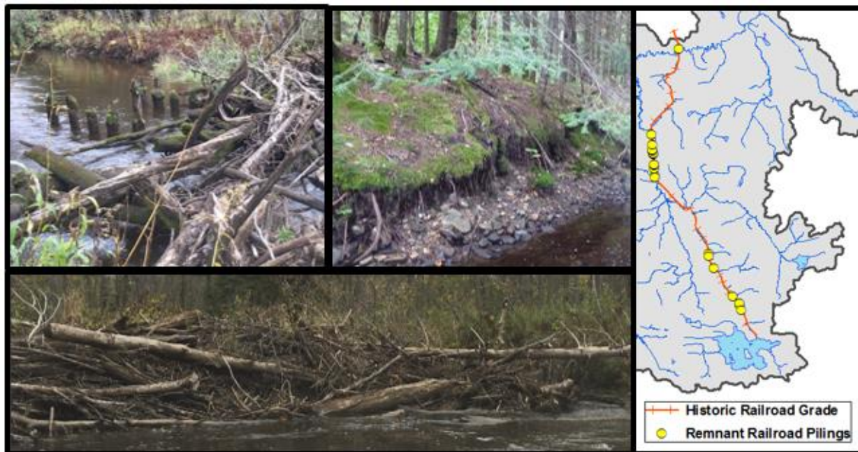
Figure 15. Map (Right) identifying locations where the old railroad historically crossed the Ash and Blackduck Rivers including one location on the Ash River and 18 on the Blackduck River. Pilings remain in the stream at many of these historic crossings causing debris pile-ups (top left and bottom). Bank erosion was identified in the Blackduck River in areas where the old railroad runs parallel with the Blackduck River (Top center).
