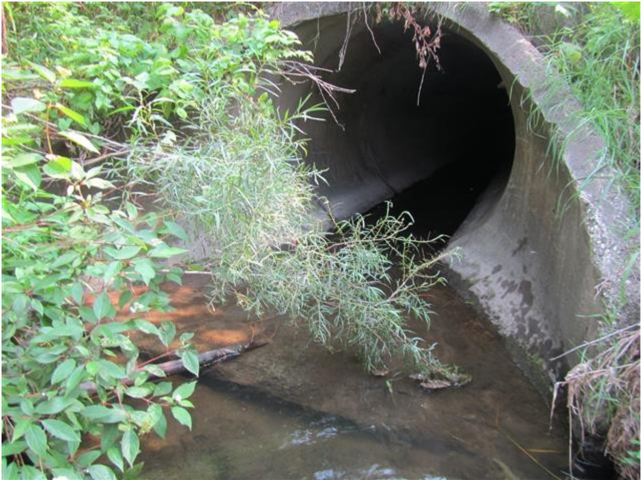
Figure 8: Picture of culvert at road crossing on 200 th Street SE on County Ditch 23, showing less than 0.10 feet of water.
