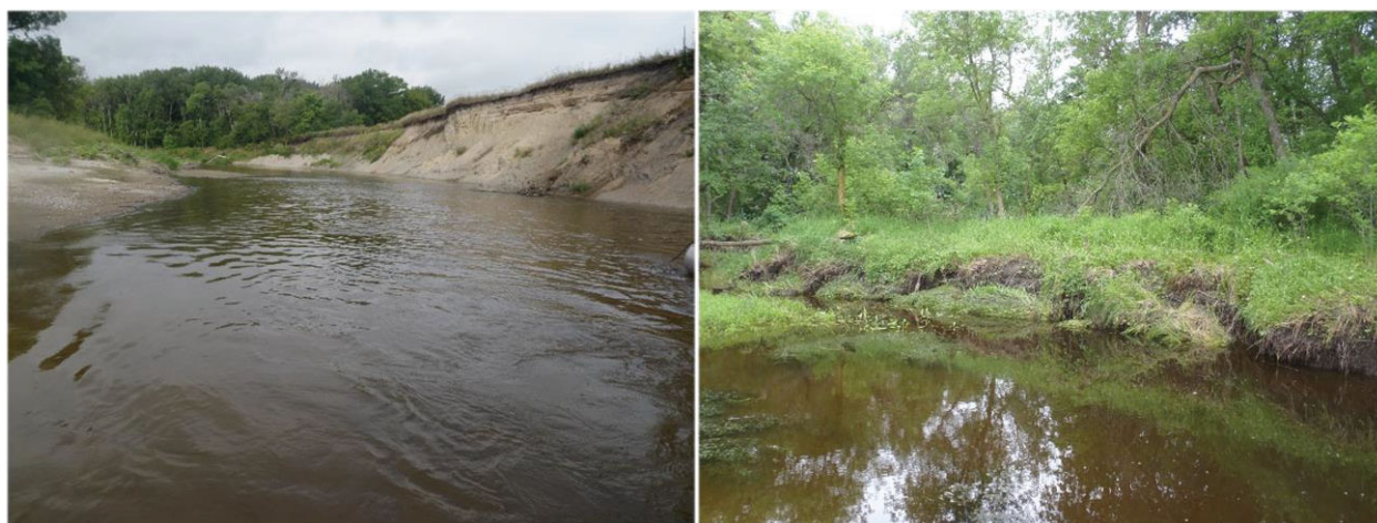
Figure 24. Images of bank instability along AUID 650, including Station 95RD014 on August 21, 2014 (left) and Station 14RD034 on June 24, 2014 (right).
