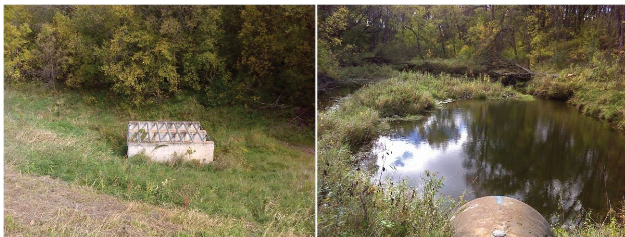
Figure 21. Images of the Mashaug Creek No. 10 Dam on September 28, 2016, including the intake structure (left) and the outflow pipe (right).
