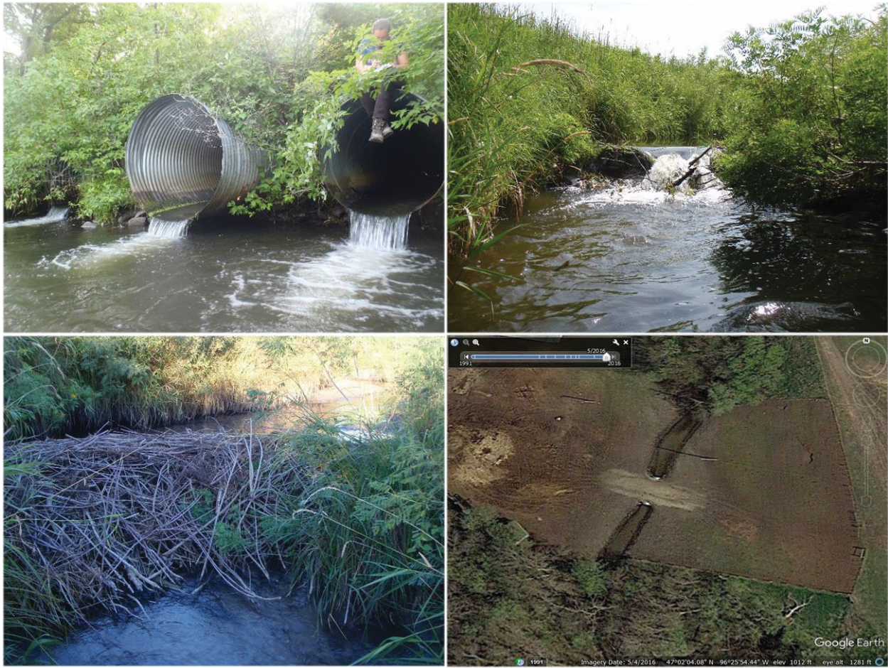
Figure 38. Images of connectivity-related issues associated with AUID 654, including perched culverts at the 170 th Street North crossing on August 7, 2014 (upper left); the remnants of a beaver dam at Station 14RD046 on August 5, 2014 (upper right); a beaver dam at Station 15RD035 on September 8, 2015 (lower left); and a private road crossing upstream of the 170 th crossing on May 4, 2016 (lower right), courtesy of Google Earth.
