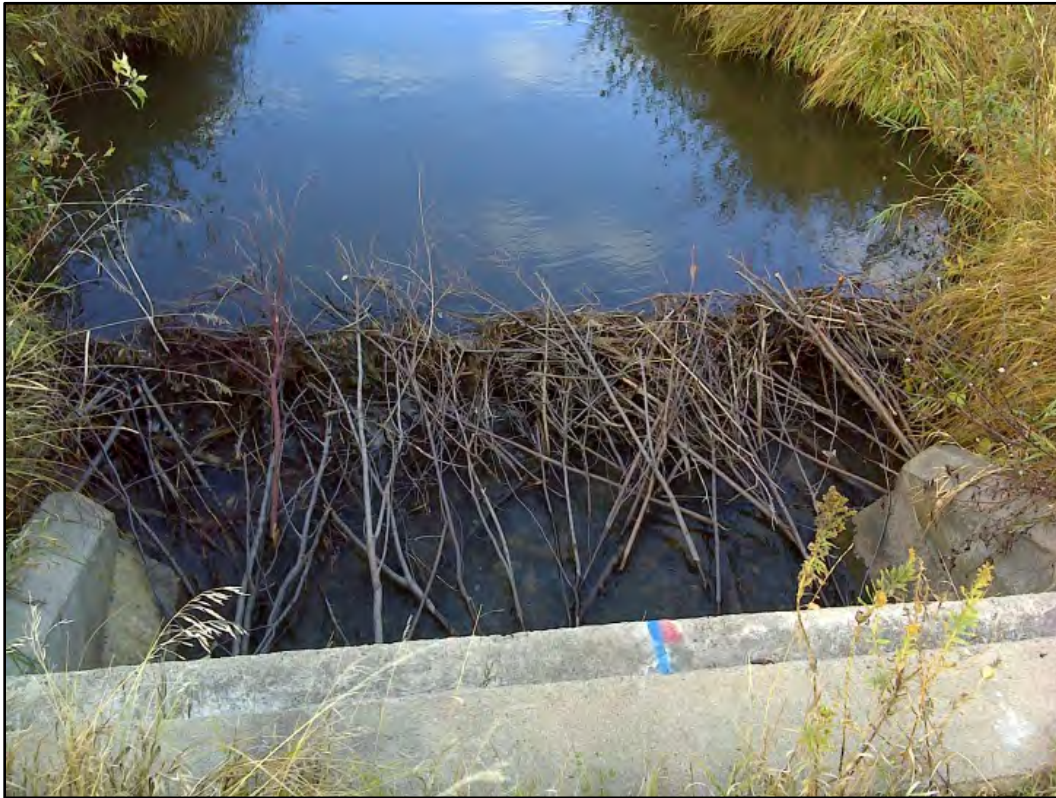
Figure 78. Beaver dam across the inlet of a box culvert found in the Upper Buffalo River.
