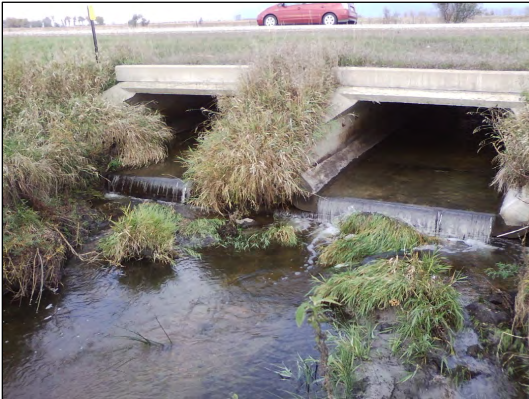
Figure 97. Photo of Deerhorn Creek at the downstream end of box culverts under Wilkin County Hwy 52.
