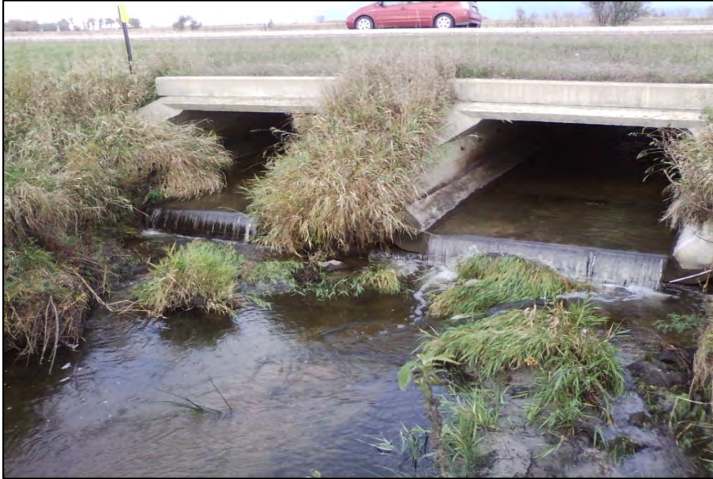
Figure 68. A perched culvert on Deerhorn Creek prevents the upstream migration of fish during low to moderate flow conditions.
