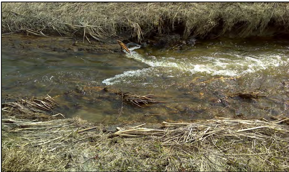
Figure 69. A head-cut in the Buffalo River system works its way upstream by eroding the stream bed.
