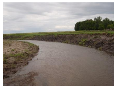
Figure 134. Severe bank erosion at site 14DM047.
