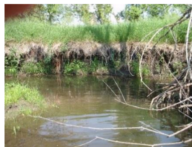
Figure 200. Bank erosion at site 14DM089.
