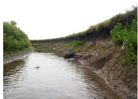
Figure 104. Severe bank erosion at site 14DM037
