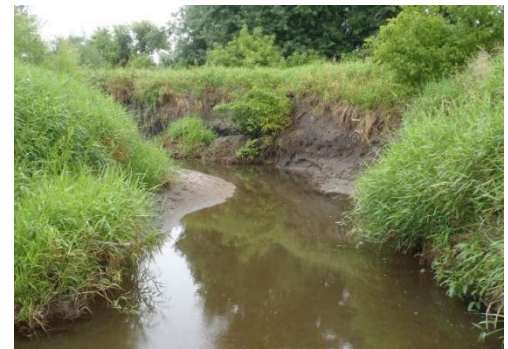
Figure 118. Severe bank erosion at site 14DM039
