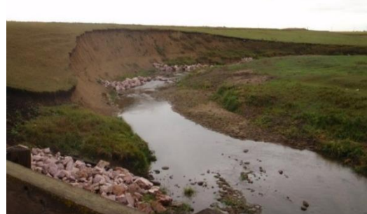
Figure 146. Severe Bank erosion at 04DM041
