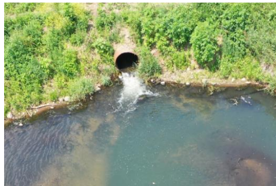
Figure 4: Perched culvert in North Creek preventing fish migration.
