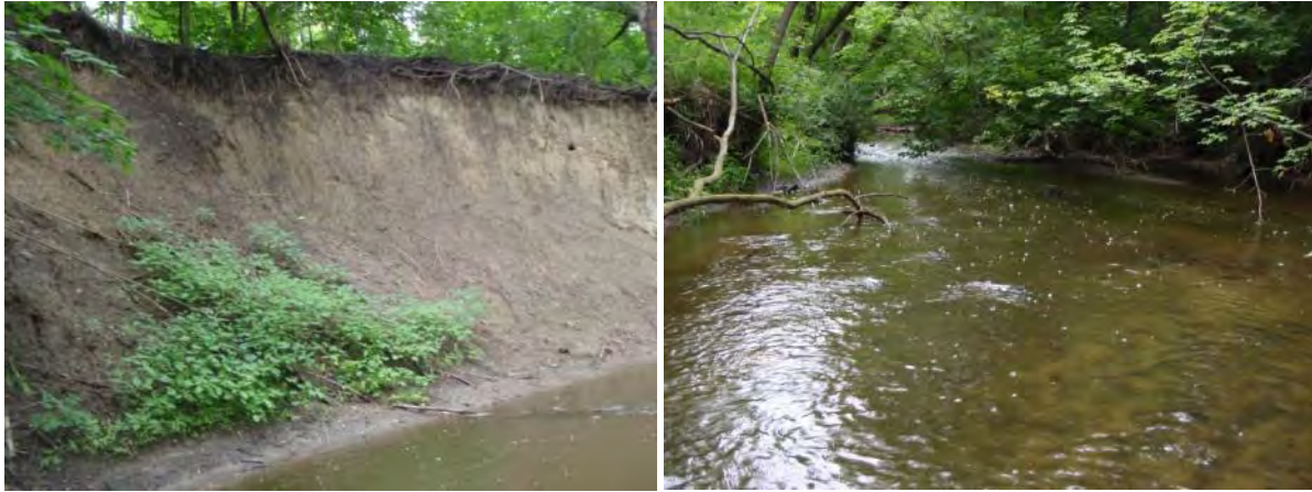
Figure 46. Photographs of station 08MN032 left bank showing heavy erosion (right) and view of reach from downstream end looking upstream (left)
