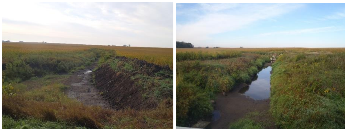
Figure 251. Biological station 13MN137 (September 12, 2012) dry streambed and small buffer (left); biological station 13MN139 (September 12, 2013) intermittent flow (right).
