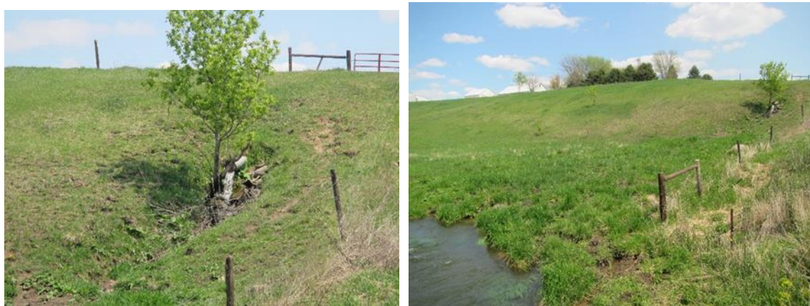
Figure 131. Biological station 13MN124 (May 2, 2016) constantly flowing pipe (left and right).
