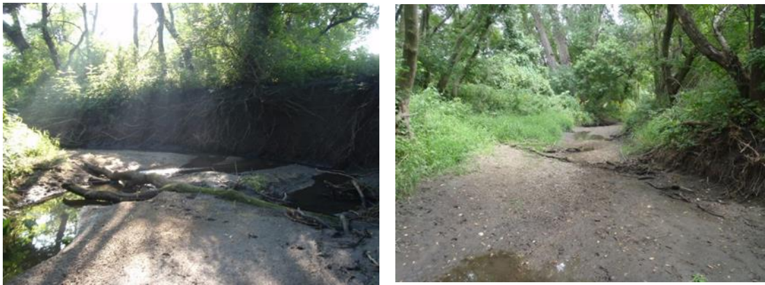
Figure 115. Biological station 13MN125 (August 15, 2013) stream bank erosion (left); low flow (right).
