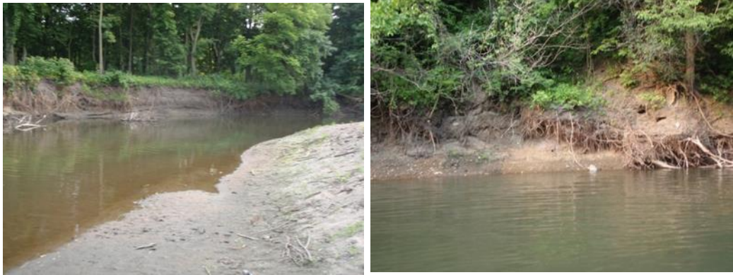
Figure 277. Biological station 13MN162 (August 12, 2013) stream bank erosion and sediment deposition (left); stream bank erosion (right).
