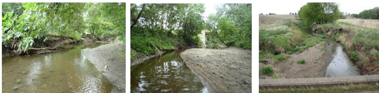
Figure 113. Biological station 13MN109 (July 2013) stream bank erosion (left); sediment deposition (middle); (May 1, 2014) sediment deposition and stream bank erosion (left).
