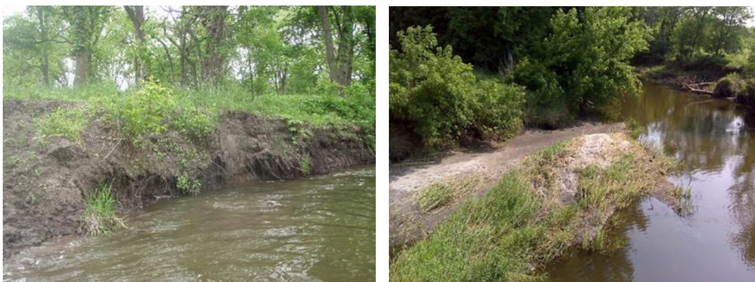
Figure 256. Biological station 97MN011 (June 10, 2013) stream bank erosion (left); biological station 01MN015 (July 10, 2014) sediment deposition (right).
