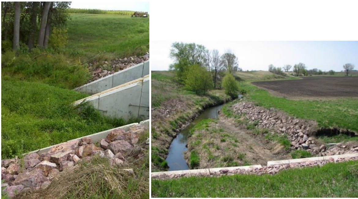
Figure 68. Biological station 13MN123 (August 27, 2015) culvert filled with sediment vegetation growing (left); (May 1, 2015) drain tile culvert caving in (right).
