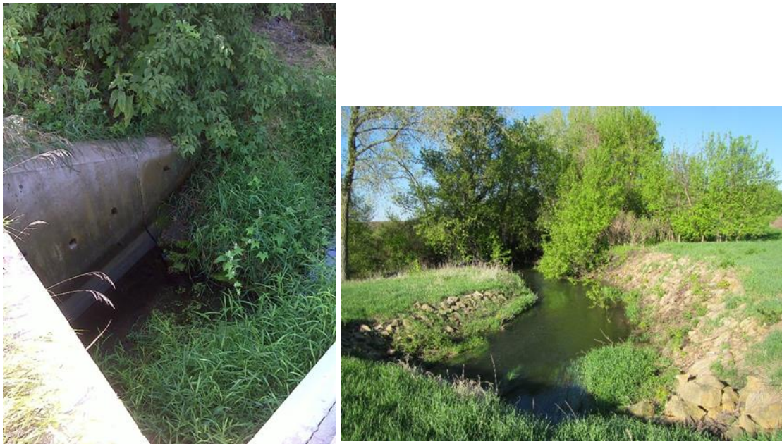
Figure 286. Biological station 13MN120 (September 1, 2015) sediment deposition in the culvert (left); (May 2, 2016) armored stream banks (right).
