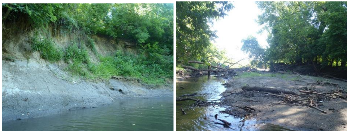
Figure 262. Biological station 13MN145 (July 19, 2013) stream bank erosion (left); (August 27, 2013) sediment deposition (right).
