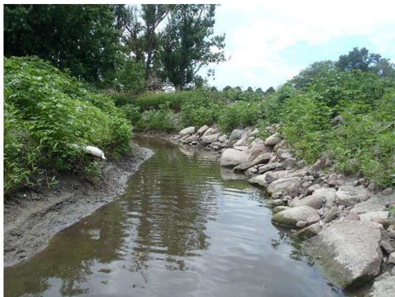
Figure 167. Biological station 13MN164 (July 23, 2013) drain tile, riprap armored bank.
