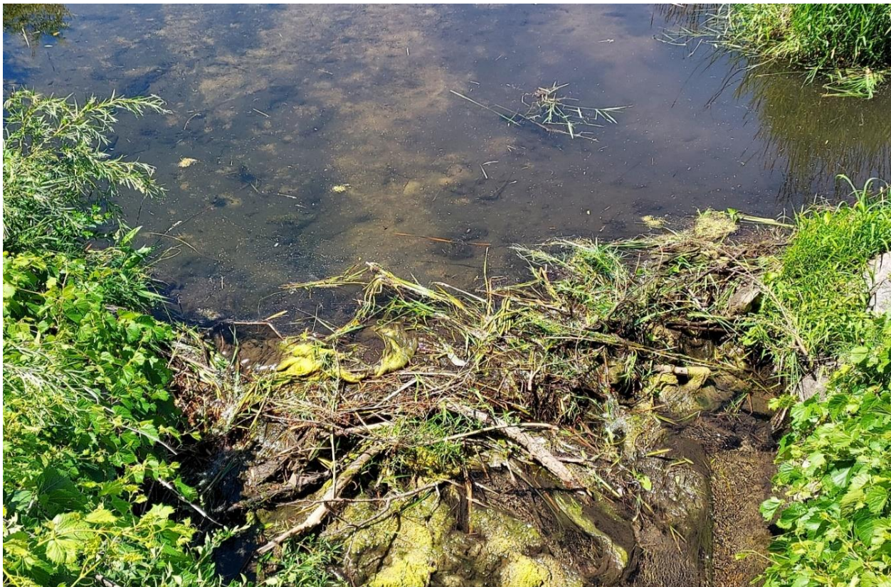
Figure 33. Culvert just downstream of bio site 09MN027 showing a likely fish barrier.
