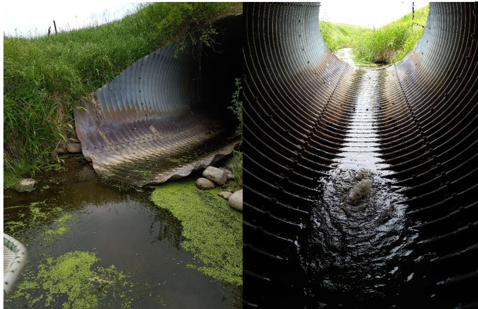
Figure 47. Photos of a culvert near bio site 09MN043. The culvert is not set at the proper elevation, creating a fish barrier.
