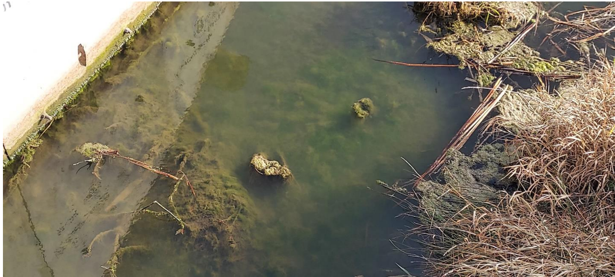
Figure 61. Culvert downstream of both bio sites showing excessive algae growth along the entire bottom.
