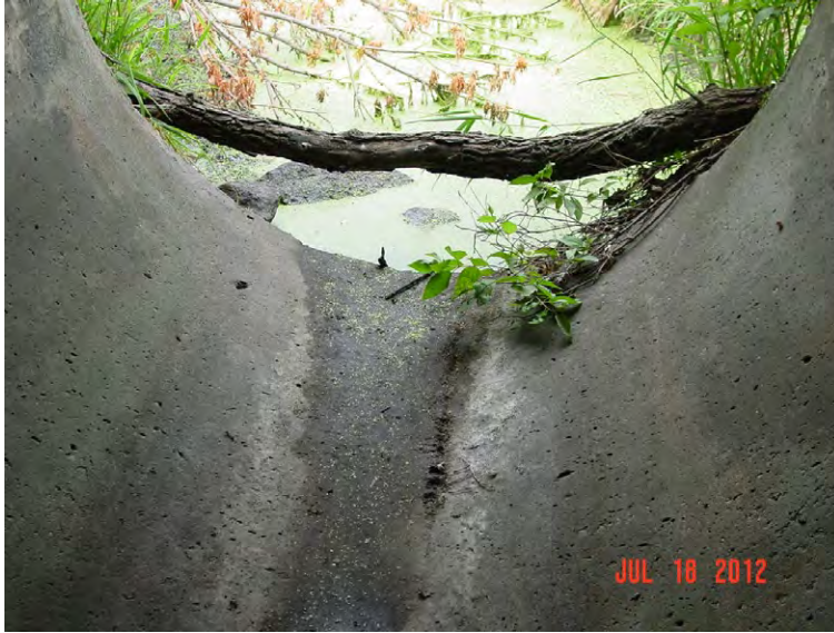
Figure 35. Dry and perched culvert in County Ditch 36 (photo taken by Hawk Creek watershed project).
