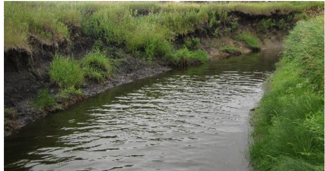
Figure 18. Bank erosion on Drywood Creek
