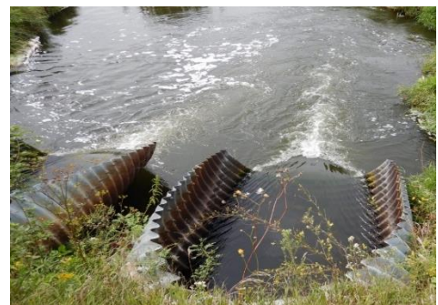
Figure 6. Perched culverts on Pelican Creek
