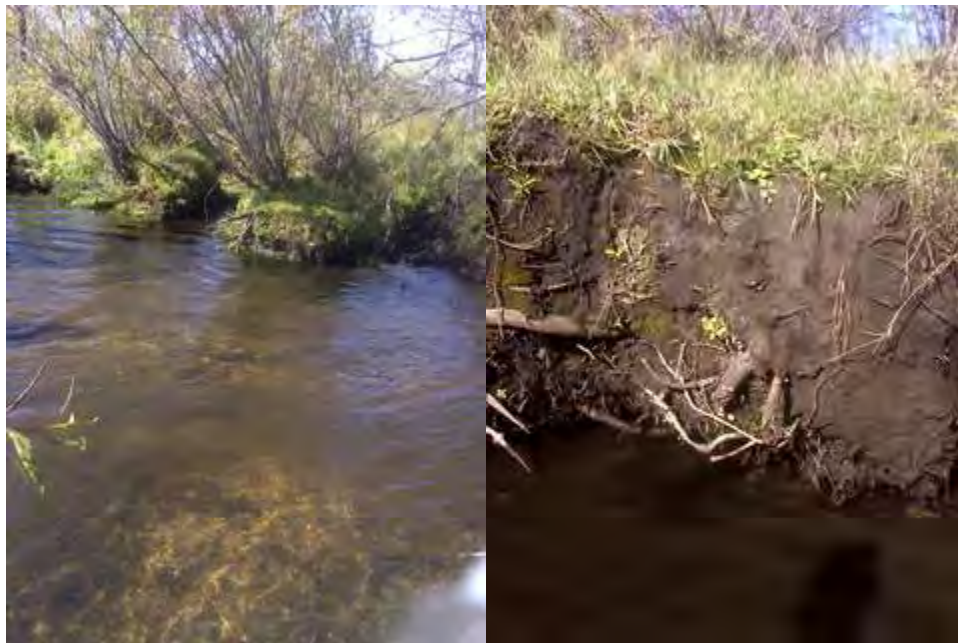
Figure 4.1.7: South Bluff Creek, photo on the left shows the fine sediment deposited on the stream bed. Photo on the right shows the stream bank eroding with a lack of deep rooted vegetation on the bank. Bank root density is low and stream banks are susceptible to erosion.
