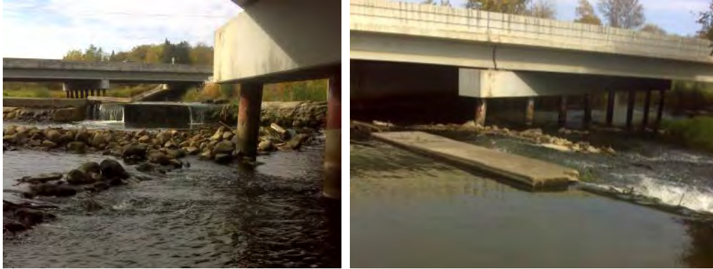
Figure 4.3.6: Dam on the Wing River located at the intersection of Highway 210 and Highway 71 in Hewitt, Minnesota. The photo on the left is looking upstream toward dam. Photo on right is looking downstream at dam. 10/2/2013 date of photos.
