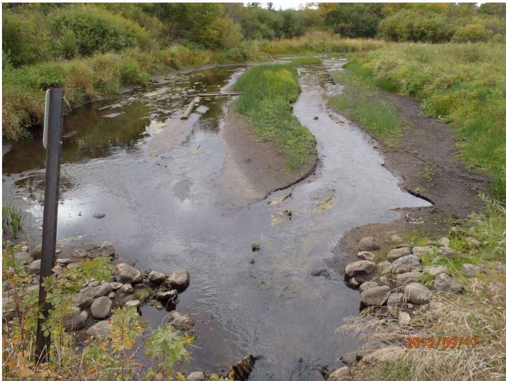
Photo 25. Sediment deposition just above the Guyles Road culvert
