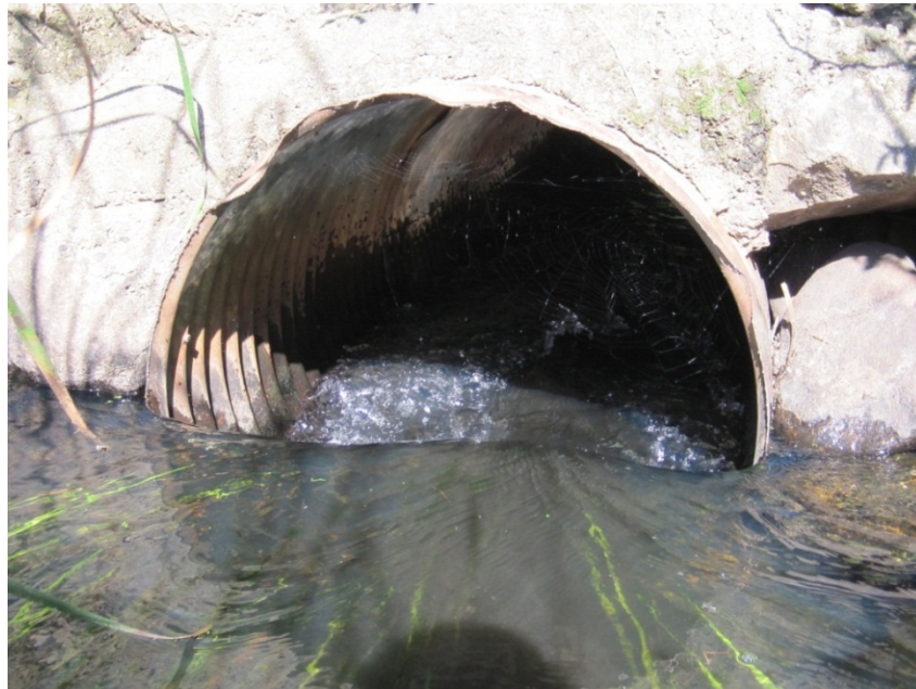
Photo 5. Upstream entrance to the Aspen Lane culvert. The culvert elevation is not correct, and it is also undersized, causing the flow to be quite swift.
