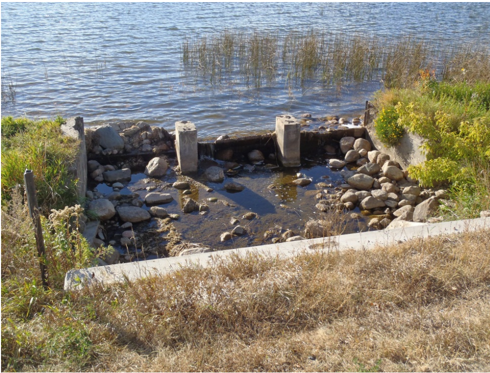
Photo 16. The small dam at outlet of Shell Lake (beginning point of AUID - 537) in fall 2012 - blocks fish movement between the lake and river, possibly restricting access to winter refuge habitat
