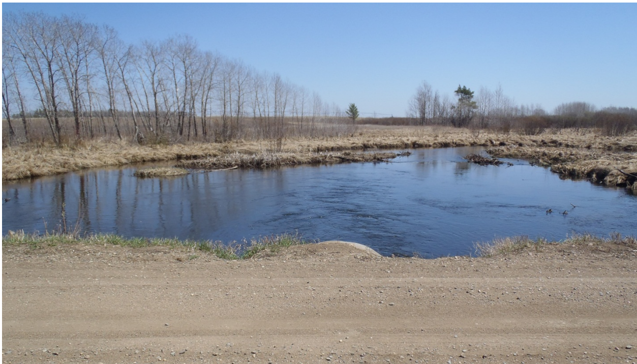
Photo 20. Culvert at 520 th Ave. Strong velocity was observed coming from the culvert, which is undersized, and this large scour pool is the result of these more-erosive flows.
