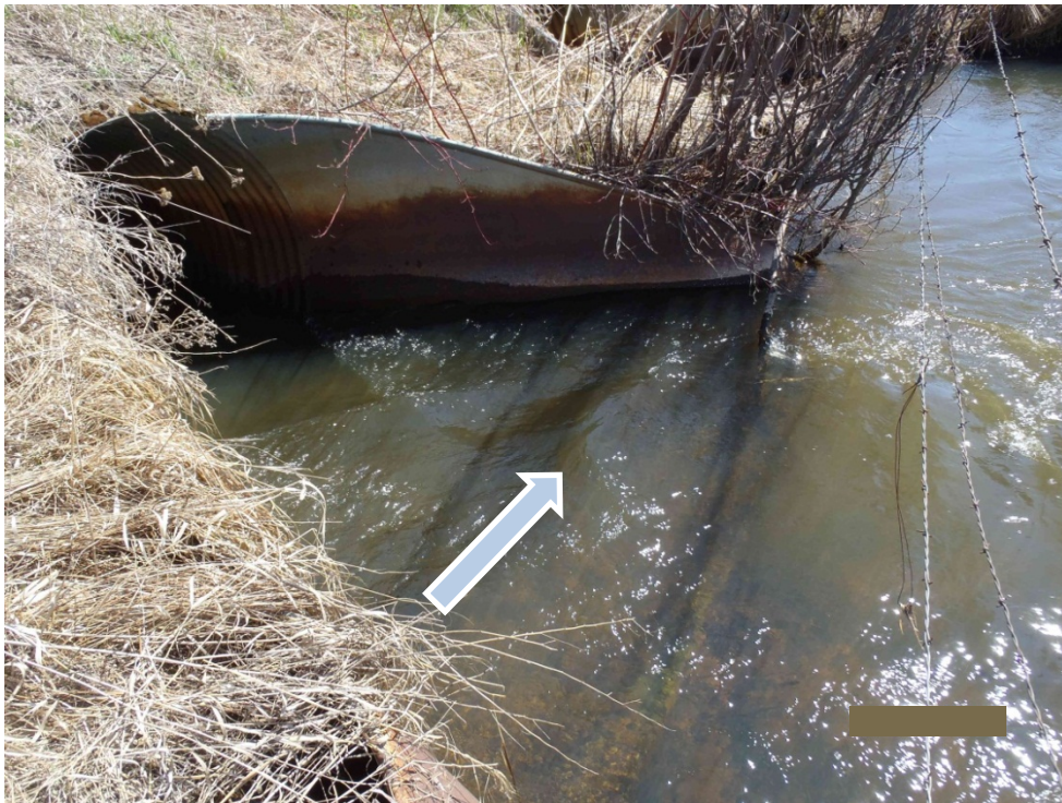
Photo 8. Outfall of right-bank culvert, May 2013. Note that even at high water, the lip of the culvert is only a few inches below the water surface. The arrow points to standing wave, a sign of high velocity.
