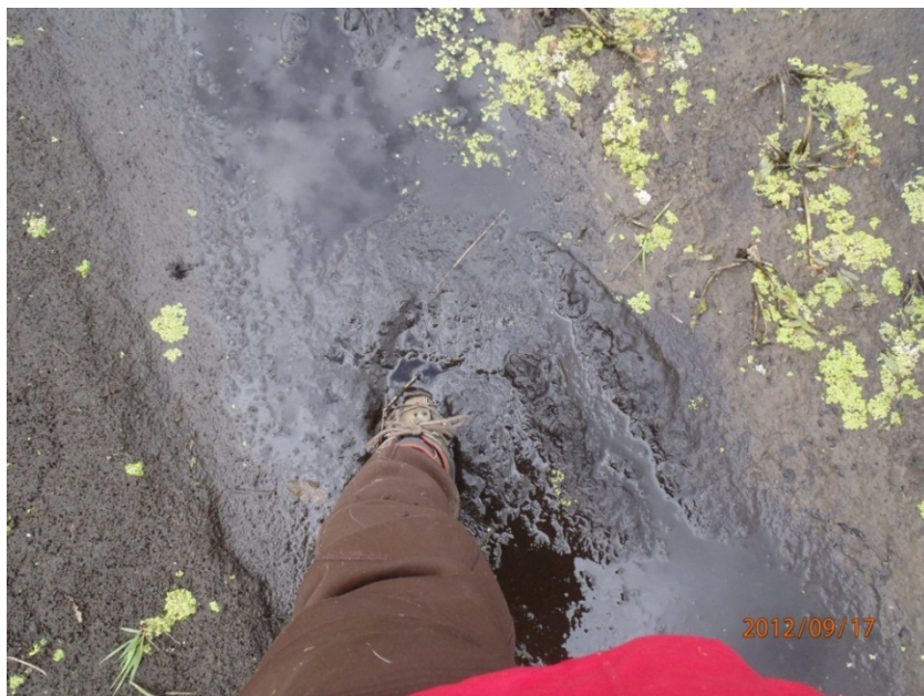
Photo 23. Muck at site 10UM053. Culvert downstream is set too high, decreasing gradient, and likely causing deposition of this organic material here. This organic sediment likely adds to the DO sag that occurs here.
