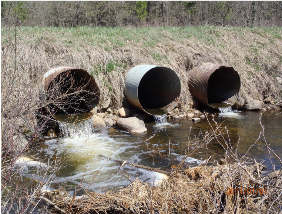
Photo 31. Perched culverts on the Blueberry River on Little Long Lake Road
