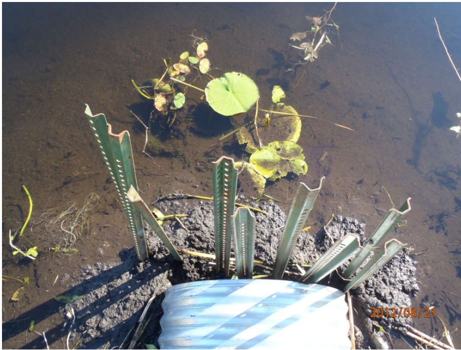
Photo 6. Outlet of Tripp Lake wetland, blocked by a mud beaver dam. There was evidence here of repeated attempts to maintain open flow in this culvert (debris pile, stakes over culvert opening).
