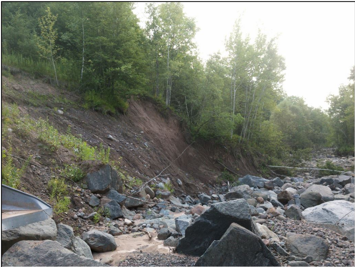
Figure 45: Severely eroding bank on the unnamed tributary to Kingsbury Creek (upper left); a ~1.0 meter headcut on the unnamed tributary to Kingsbury Creek (upper right); and major bluff erosion site downstream of HWY 2 (lower)
