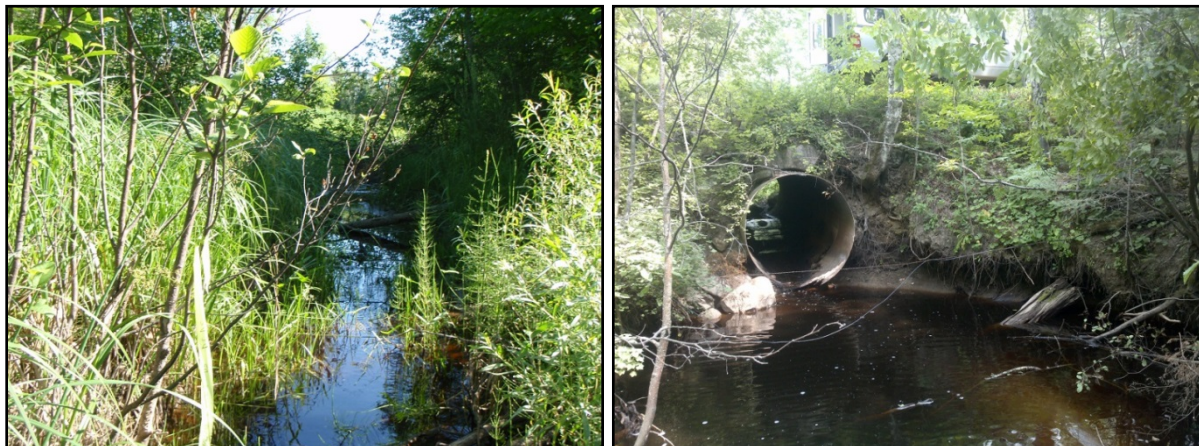
Figure 162: Photos of Unnamed tributary to St. Louis River at County Road 52. Note low flow conditions and possible barrier to fish passage (right).
