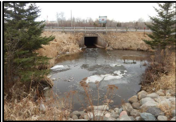
Figure 22b. Culvert on Miller Creek at US Hwy 53 crossing during snowmelt. The culvert becomes perched and acts as barrier to fish passage during the low flow season. The plunge pool downstream is an indication of an undersized culvert.
