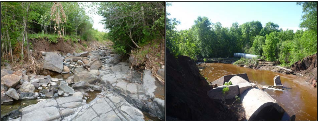
Figure 48: Streambank and infrastructure damage along Kingsbury Creek caused by extreme flood event in June 2012.
