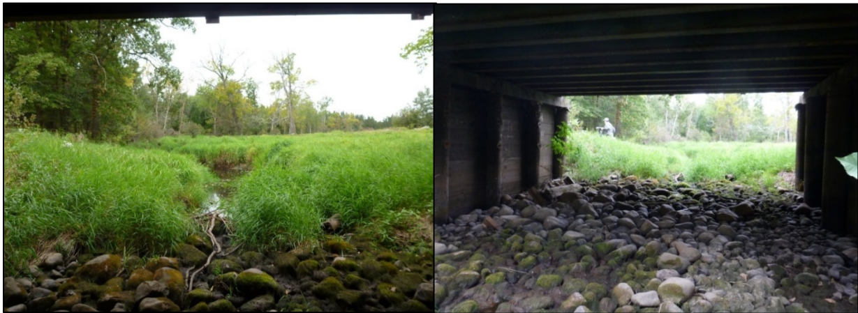
Figure 112 (Left): Looking upstream from CR 196 bridge. The cobbles added during bridge construction were set at too high of an elevation. Water flows subsurface through cobbles, and the improper crest elevation of the cobbles is creating a flat water surface upstream. (Right): The coarse cobble substrate and lack of water underneath the CR 196 bridge.
