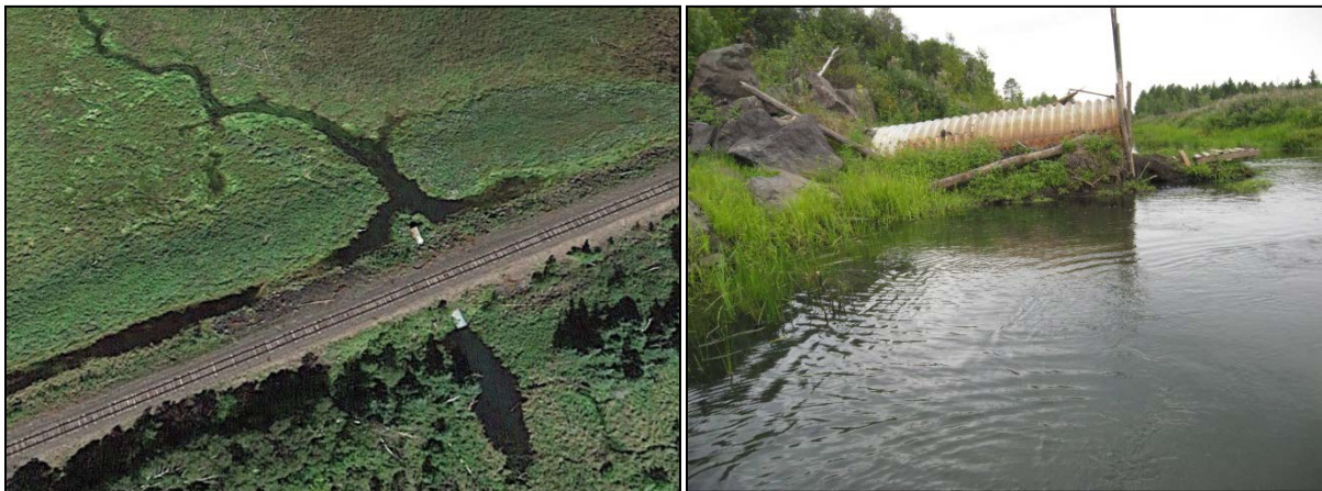
Figure 209: An example of a connectivity issue on Wyman Creek. This culvert is perched, degraded, and filled with sediment and large wood which reduces or eliminates
