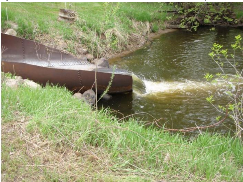
Figure 62. Perched culvert on Rice Creek off 57 th St. SE, Sherburne County
