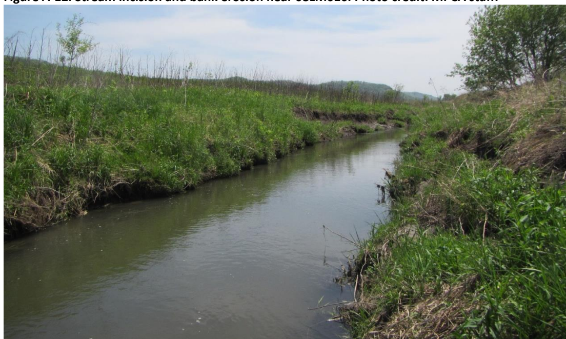
Figure A-12. Stream incision and bank erosion near 08LM016. Photo credit: MPCA staff.
