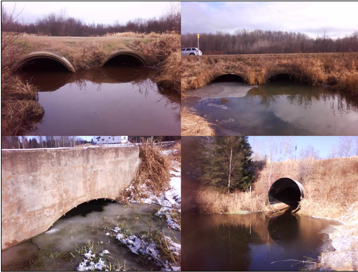
Figure 24: Examples of inadequate capacity (above right, above left, and bottom left) and a scour pool caused by an overly narrow culvert
