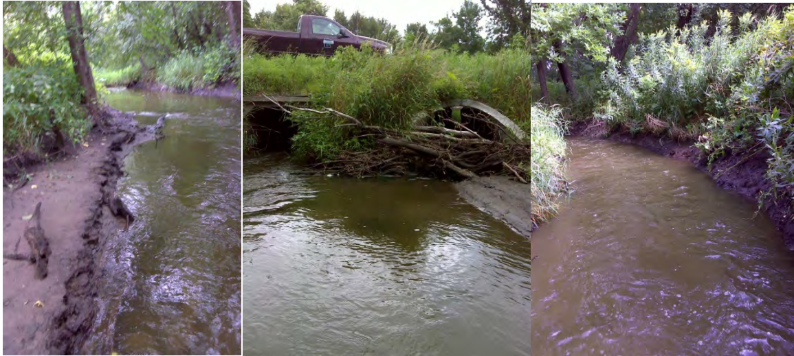
Figure 99: Typical bank condition on Unnamed Creek upstream from Nabor Avenue. Note the debris on culvert. Storm flows are cleaning out the channel moving any beneficial woody debris downstream. Note the brown color of stream on right photo.
