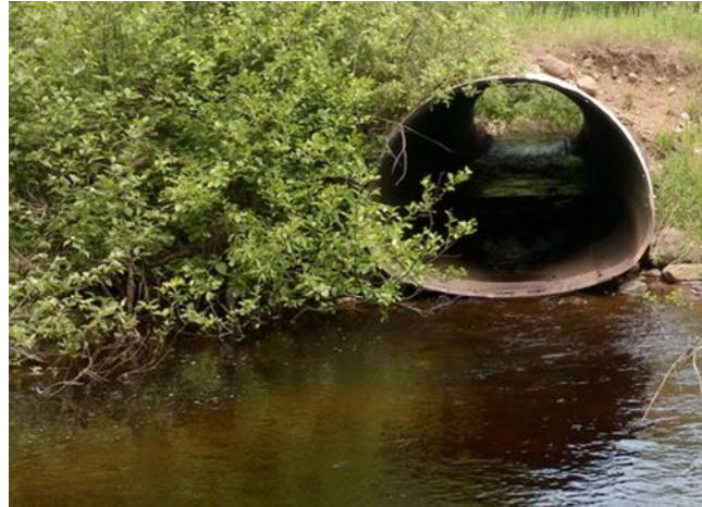
Figure 7. A perched culvert disrupting flow and fish passage in a stream
