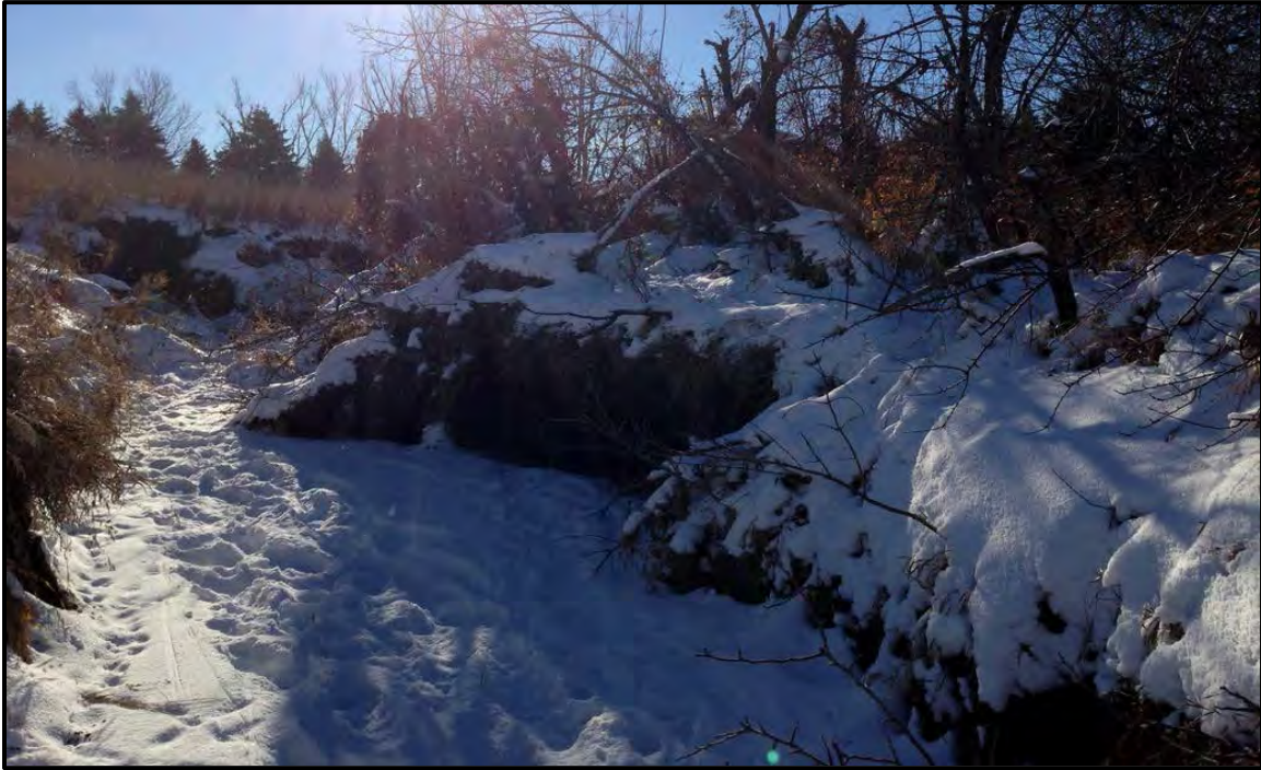
Figure D-7. Sunset Bay tributary streambank erosion location SB3L.
