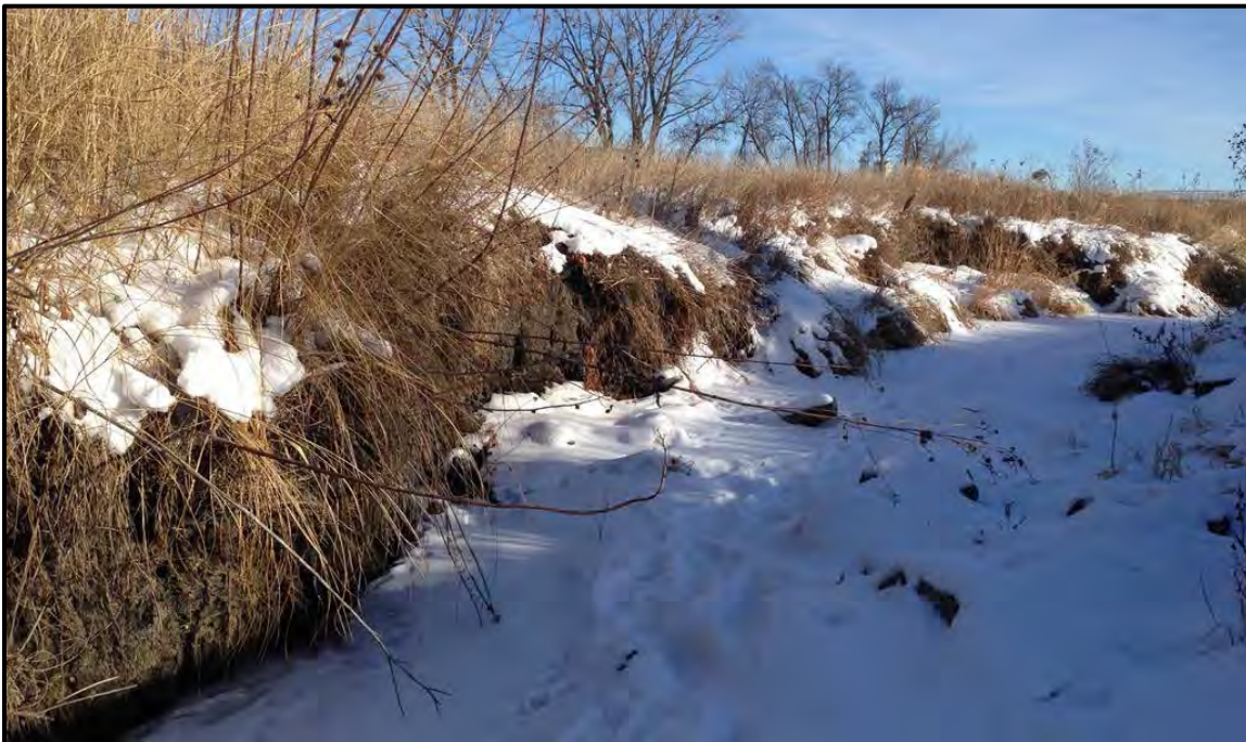
Figure D-2. Okabena Creek streambank erosion location OKA12.
