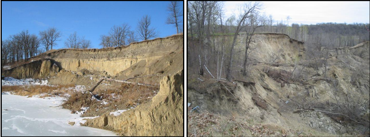
Figure 4-3. Photos of eroding bluffs along the Red Lake River near Red Lake Falls.
