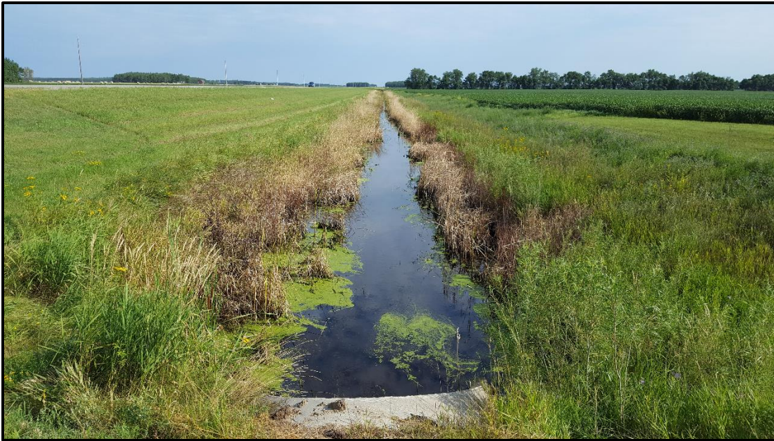
Figure 4-42. Photo of the Pennington County Ditch 43 Channel (09020303-547). The trapezoidal channel geometry and the results of weed spraying activity can be seen in this photo.
