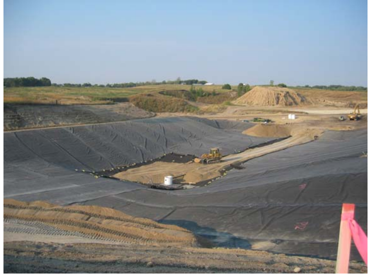
Liner Construction at Otter Tail Power Company's Hoot Lake Landfill. Photo by Kathy Holland-Hanson
