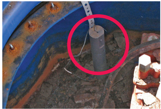
Photo 6: Examples of sump sensors.
