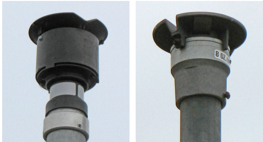
Photo 14b: Close up of the pressure vacuum vent covers.
