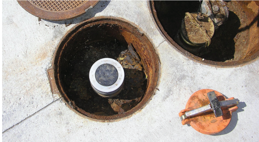
Photo 13: Dual point vapor recovery. Vapors are recovered from the riser on the left. A probe cover sump is on the right. A ballfloat is the overfill protection.
