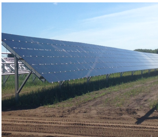
First Solar thin film modules were selected for the 10-megawatt solar photovoltaic power plant. These advanced thin film modules have a demonstrated performance advantage over conventional crystalline silicon of up to 10% more energy production each year. Source: MN National Guard Public Affairs Office
