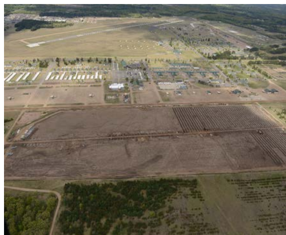
Construction of the 10-megawatt solar photovoltaic power plant spans 62 acres on a former gravel mining pit at Camp Ripley Training Center.
