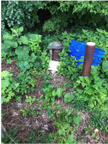
Photo 19 MG-2. 8-10" steel outer casing, Two bollards one with electrical box attached, don't appear damaged.
