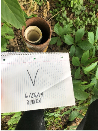
Photo 7 Well V. 2" PVC well casing, no well plug, one bollard, appears to have old/abandoned well or broken bollard behind it.
