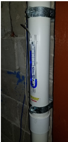
Photo 29- Varsity Apartment- commercial system.
