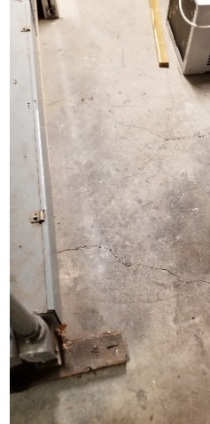
Photo 32- Cracks in floor at Varsity Apartments.
