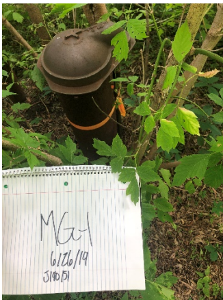
Photo 3 Well MG-1. Hidden under vegetation and behind a tree. Two bollards present, one appears to have been backed into and is slightly bent.
