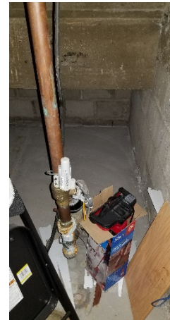
Photo 28 Varsity Apartment- commercial system.
