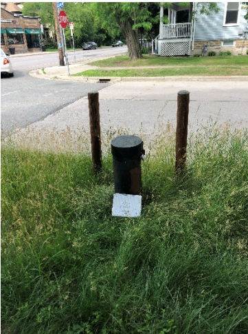
Photo 9. Well 200. 8-10" steel outer casing, two bollards on road side, pumping housing and electrical plug inside well. No damage noted.
