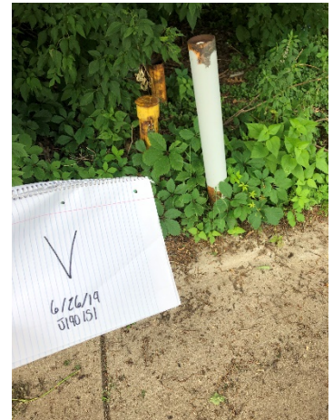
Photo 30- 2" PVC well casing, no well plug, one bollard, appears to have old/abandoned well or broken bollard behind it.
