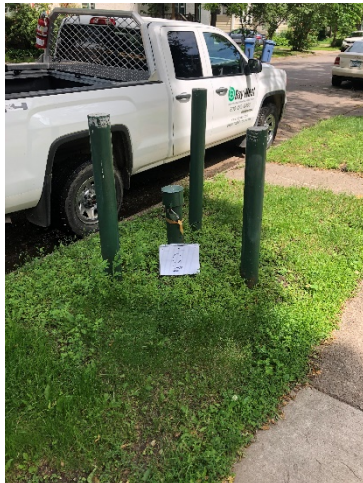
Photo 21- Well Q. 2" PVC well casing, plug present, three bollards. No apparent damage.
