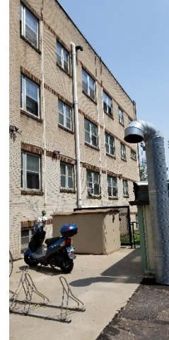
Photo 26- Varsity Apartment- commercial system.
