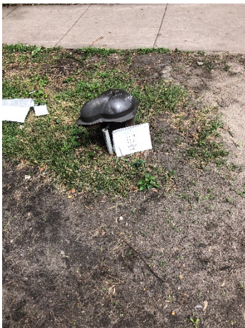
Photo 5 Well 112. 8-10" steel outer casing, electrical wires protected by PVC piping outside of well, cap bolted on, did not open. No bollards.
