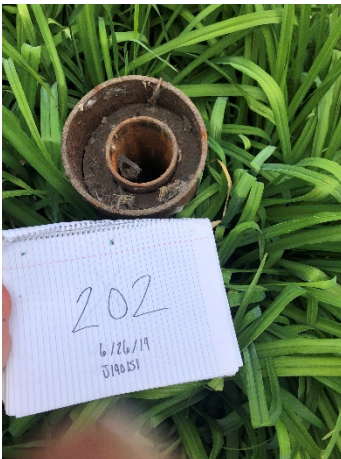
Photo 11 Well 202. 4" steel well casing, surrounded by vegetation, no plug/cap, no bollards.
