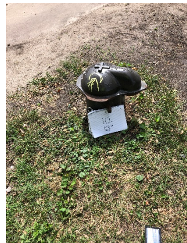
Photo 6 Well 112. 8-10" steel outer casing, electrical wires protected by PVC piping outside of well, cap bolted on, did not open. No bollards
