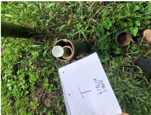
Photo 27- Well T. ~2" PVC well casing, plug/cap present, three bollards. No apparent damage.
