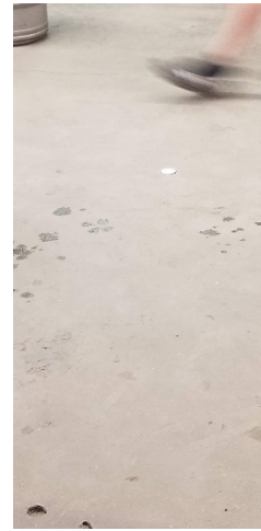
Photo 8 Sub slab vapor pin in Building 10.
