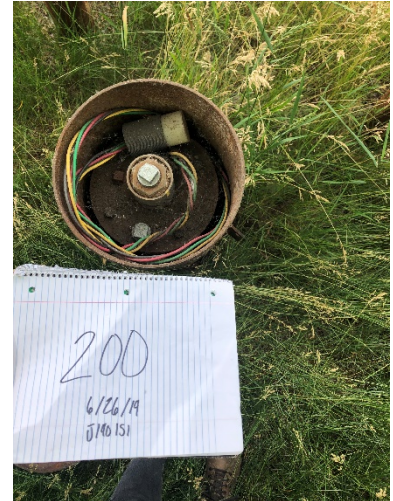
Photo 8 Well 200. 8-10" steel outer casing, two bollards on road side, pumping housing and electrical plug inside well. No damage noted.
