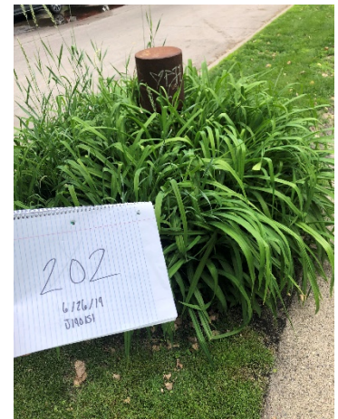
Photo 12 4" steel well casing, surrounded by vegetation, no plug/cap, no bollards.
