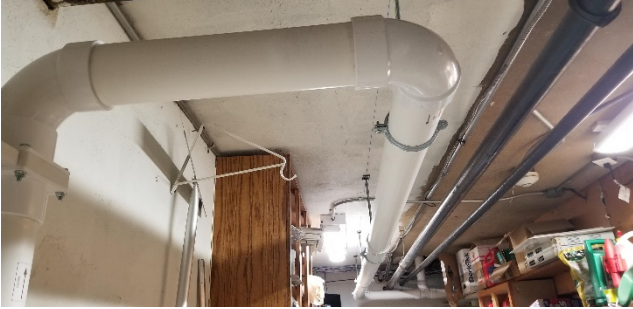
Photo 31- Varsity Apartment- commercial system.
