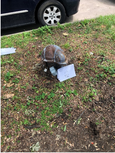
Photo 7 8-10" steel outer casing, electrical box attached to outside of well, appears slightly damaged. Cap bolted on, did not open, No bollards.
