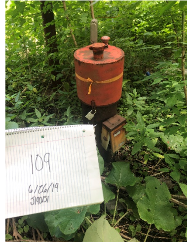
Photo 2- Well 109 In wooded area. Damaged electrical box attached to outside of well.
