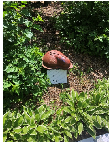
Photo 4. Well 111, 8-10" steel outer casing, electrical box attached to outside of well. Cap bolted on, did not open. No bollards.
