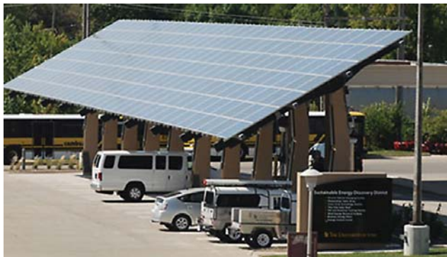
This solar e-car charging station on the campus of the University of Iowa provides charging spaces for approximately 20 electric vehicles for Facilities Management and other departments. The project was completed in summer 2011.
